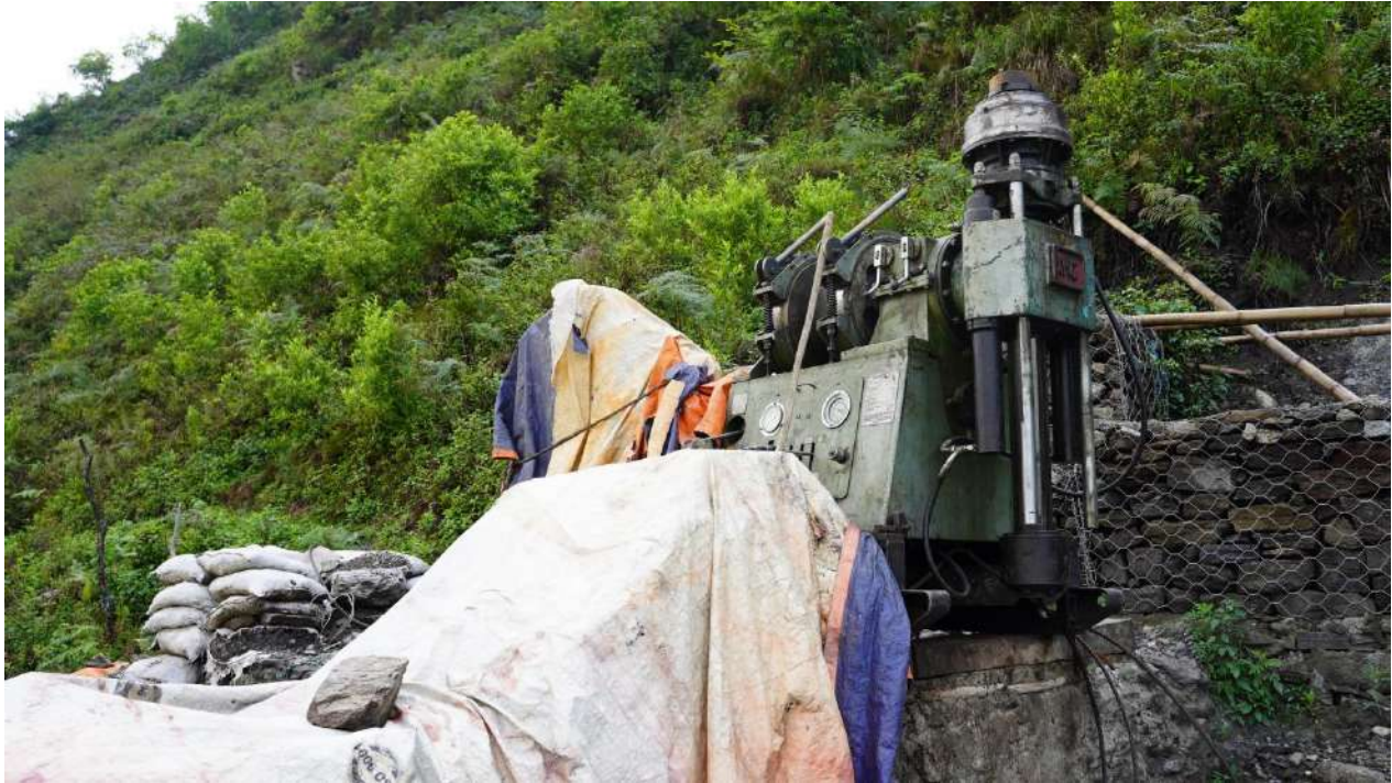
Figure 1: Drilling machine stationed towards the east of intended point of left skid contact
